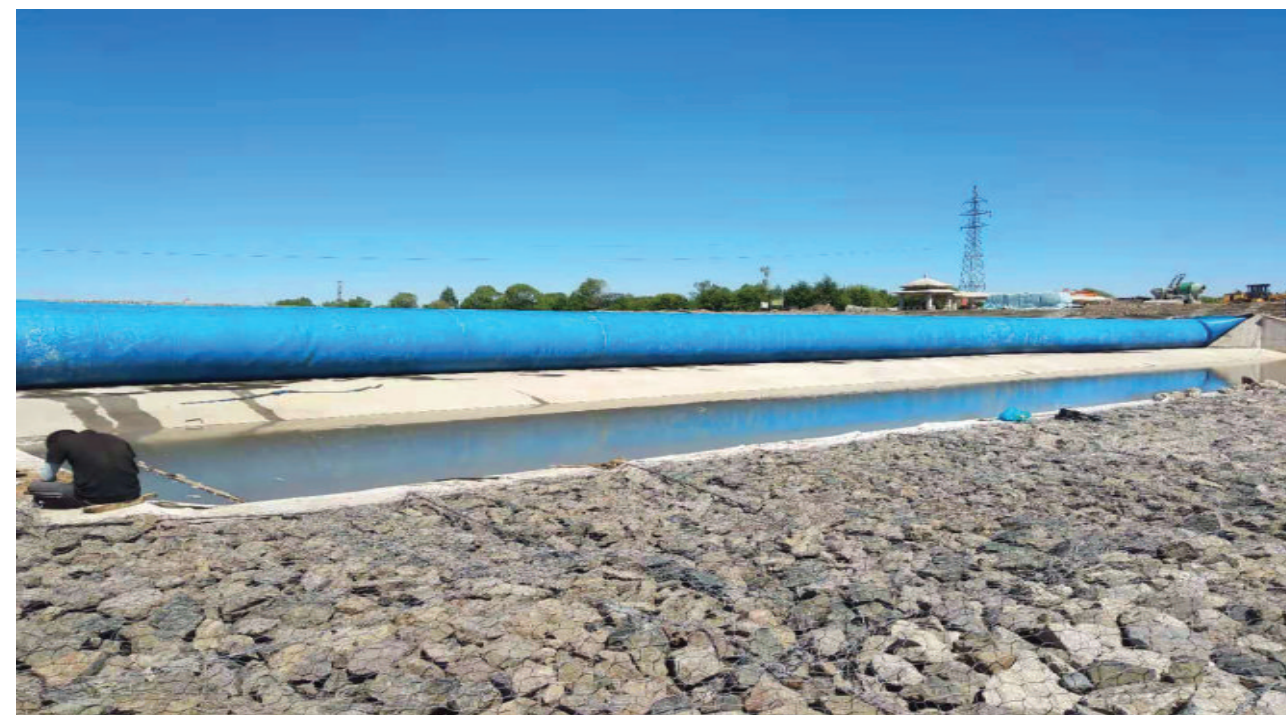
Rubber dam for sunwu Country Binshui Park, Heihe City, Heilongjiang province.
