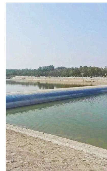
Rubber dam in Yucheng, Shandong
